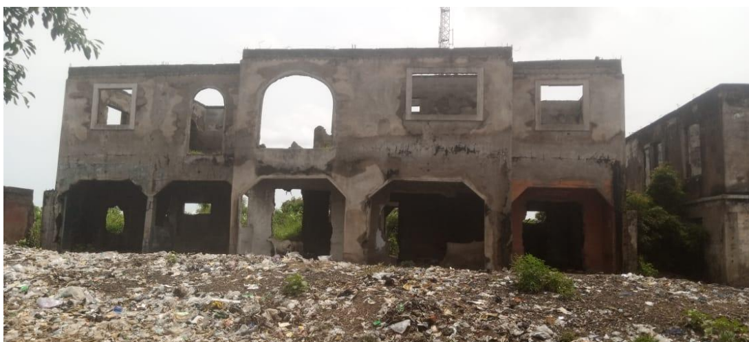
Figure 1. A burnt building in Wukari turned into a refuse dump. It symbolises total relinquishment, community neglect, and the ruin of post-crisis salvage efforts.
